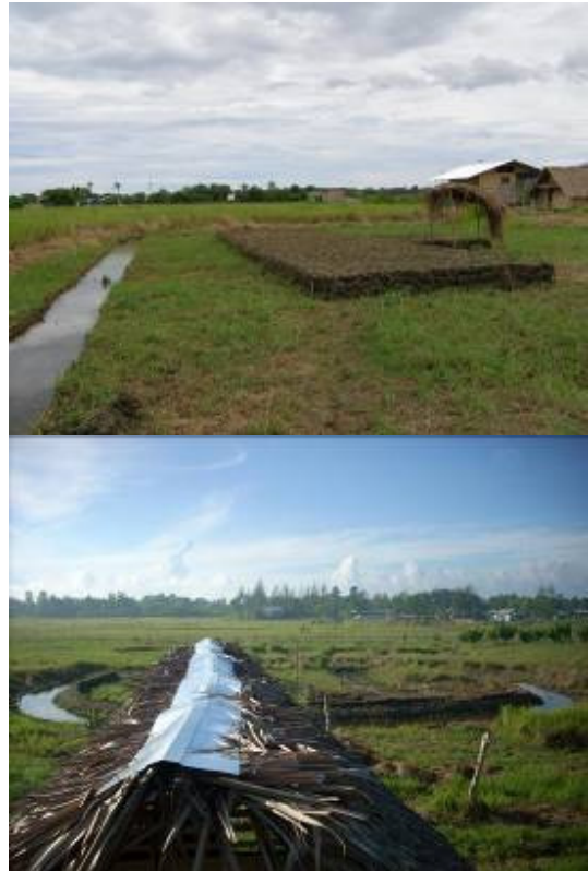
Figure 22. Manual excavations to backfill the sites for the aviary and the porcupine enclosure were completed. ©SSchoppe
